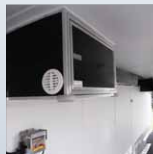
Furnace Cabinet w/Registers
