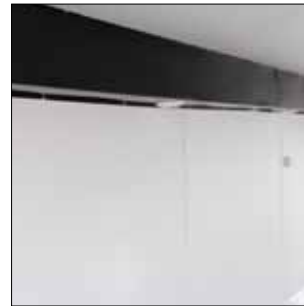
Furnace Duct with Registers
